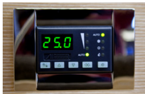
Air condition (up to 32.000 BTU) 3 units
